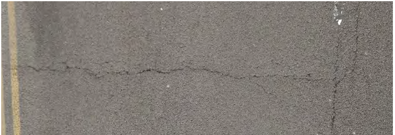
Figure 10: Transverse and Longitudinal Cracks (c)
