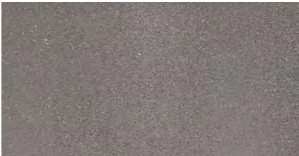
Figure 13: Loss of Aggregates/Fretting (f)
