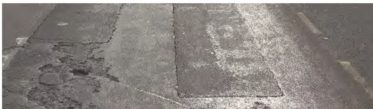
Figure 8: Loss of Aggregates (-) and Evidence of Pothole Formation (p)
