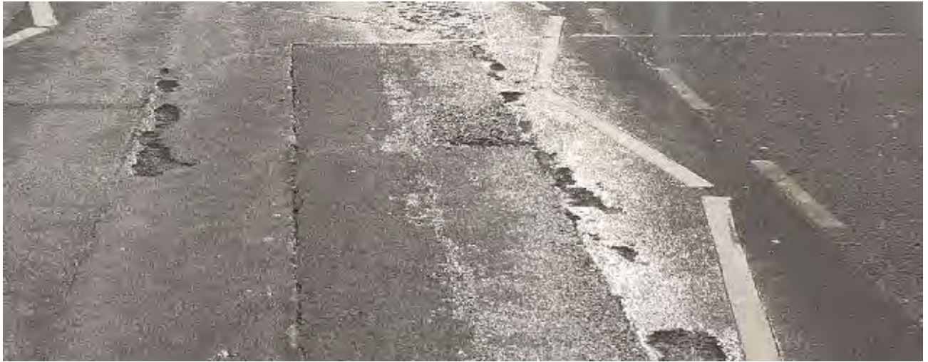
Figure 9: Variable Defects (v) including Potholes (p)
