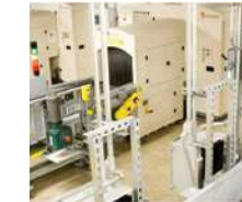
Baltimore / Washington International Thurgood Marshall Airport (BWI) Concourses D/E Baggage System and Claims Improvements, Baltimore, MD
