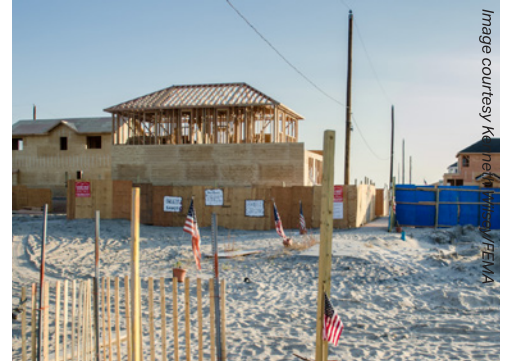
Superstorm Sandy Build-it-Back Program (NY) Provided case management for 30,000+ applicants and construction management for 1,100+ homes under a $1.4B HUD CDBG-DR-funded program
