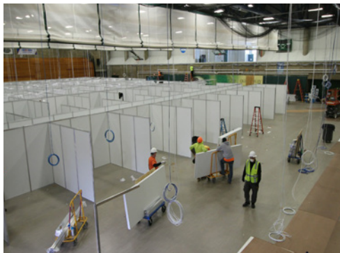
Coronavirus Response (US) Supported multiple agencies including USACE under FEMA assignments, to develop 10 alternate care and testing facilities in six states
