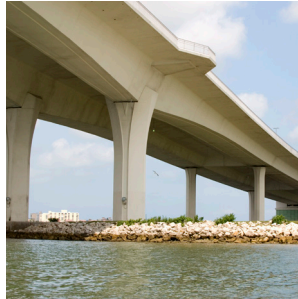
Memorial Causeway Bridge Clearwater, Florida, United States Tender design; detailed design and documentation; construction stage services 2002
