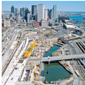
Central Artery Tunnel Project Boston, Massachusetts, United States Detailed design and documentation; construction support services 2004
