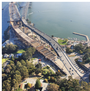
Bay Bridge East Approach San Francisco and Oakland, California, United States Structure construction engineering and inspection services 2013
