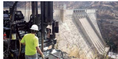
Pine Flat Dam Slope Failure Investigation and Mitigation Design Fresno County, CA
