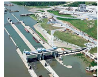
Olmsted Dam and Locks Ohio River, Illinois and Kentucky, USA We are the lead partner to construct this 2,700-foot-long concrete dam across the Lower Ohio River. The dam includes five, 110-foot tainter gates and a navigable pass section with boat-operated wicket gates. In-the-wet construction includes use of a 5,100-ton-capacity super gantry crane (pictured at top of page) to move precast concrete elements of the dam.
