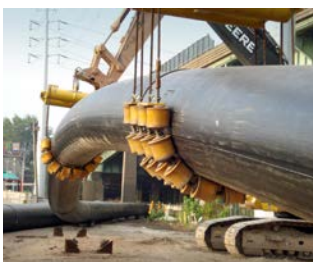
Twin Force Main Relocation Horizontal Directional Drilling Harbor Crossing New Haven, Connecticut, USA
