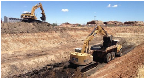
Former McClellan AFB Remediation Finished design/construction in under a year, minimizing leachate mgmt during rainy season; excavated/transported waste w/o impacts to local businesses
