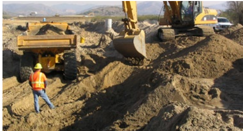
Former MCAS El Toro Environmental Remediation 20 years supporting Navy's IRP remedial design, remedial action, LTM and O&M for soil and groundwater
