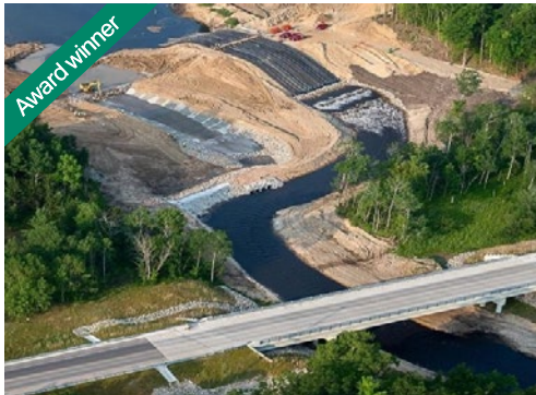
Boardman River Dam Removal (MI) On Michigan's largest river restoration project, supported USACE with work including natural channel design, structural and geotechnical analysis of dam breaching, and sediment management
