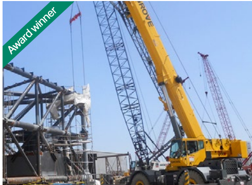
Inner Harbor Navigation Canal Protection (LA) Part of design-build team that constructed 9,000-ft surge barrier in New Orleans, preventing significant damage during future hurricanes
