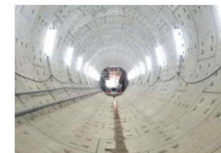
Ho Chi Minh City MRT Line 1 CP1b First metro line in Ho Chi Minh City, ø6.65 m OD EPB TBM, Vietnam
