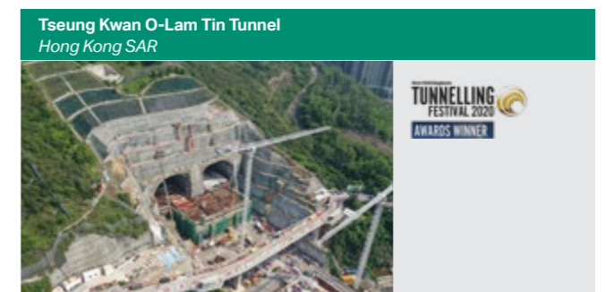
Tseung Kwan O-Lam Tin Tunnel Hong Kong SAR Large-scale semi-caverns as part of road tunnels
