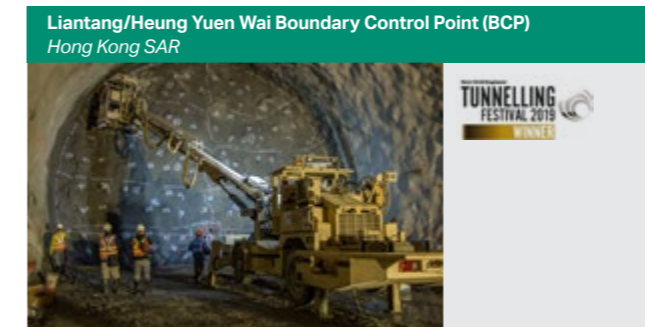
Liantang/Heung Yuen Wai Boundary Control Point (BCP) Hong Kong SAR Drill and blast, ø14.1 m OD Earth pressure balance (EPB) TBM
