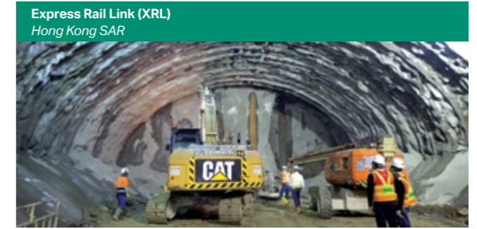
Express Rail Link (XRL) Hong Kong SAR Largest rock cover (650 m) and longest tunnel (7.6 km) in Hong Kong SAR
