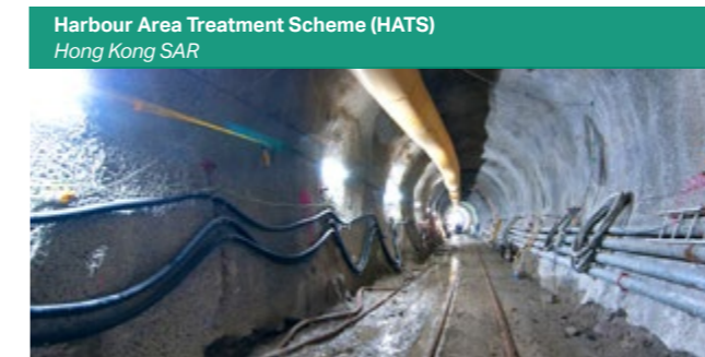
Harbour Area Treatment Scheme (HATS) Hong Kong SAR Deepest sub-sea tunnel (160 m below sea) in Hong Kong SAR
