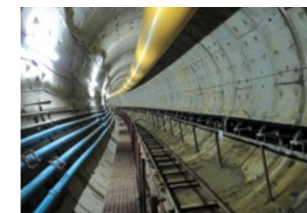
Bangkok MRT Blue Line Extension Sub-river tunnel, ø6.3 m OD EPB TBM Thailand
