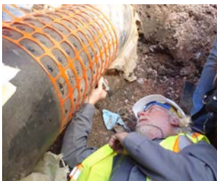
Assessment and Rehabilitation of Potable Water Mains Colorado Springs, Colorado, USA Condition Assessment Technical Practice Leader, Christopher Macey, measures the pipe thickness using ultrasonic technology equipment to estimate the remaining pipe life.
