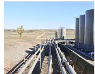
Private Water System Master Planning and Design McKenzie County, North Dakota, USA A water distribution and water disposal system plan was developed for an industrial service area covering 800 square miles/2,048 square km, including multiple pressure zones.
