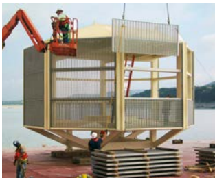
Water Treatment Plant No. 4, Raw Water Intake Screen Austin, Texas, USA
