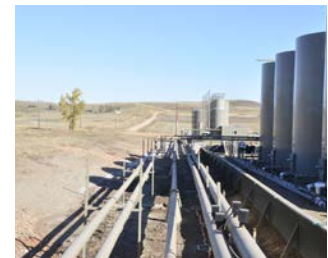
Private Water System Master Planning and Design McKenzie County, North Dakota, USA A water distribution and water disposal system plan was developed for an industrial service area covering 800 square miles/2,048 square km, including multiple pressure zones.
