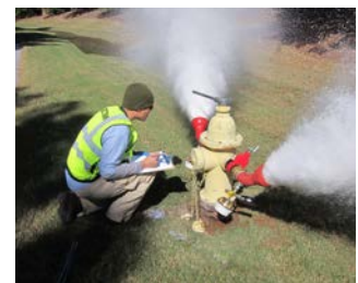
DeKalb County Water and Wastewater Capacity Master Plan DeKalb County, Georgia, USA Flow and pressure tests are performed to assist with calibration of water distribution system models.
