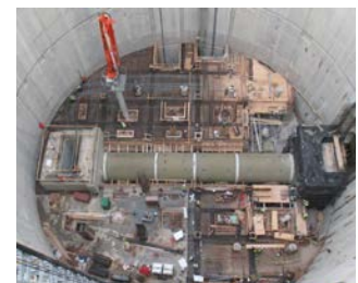
Tunnel Dewatering Pump Station Washington D.C., USA
