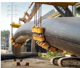
Twin Force Main Relocation Horizontal Directional Drilling Harbor Crossing New Haven, Connecticut, USA
