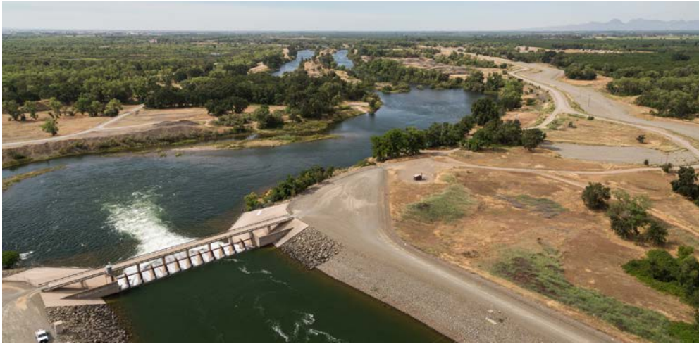
Feather River West Levee Yuba City, California, USA Thirty-five miles of 80- to 120-foot deep open trench and deep mixing method cutoff walls were installed along the Feather River West Levee
