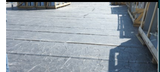
Moisture has created wrinkles and bubbles on this fully adhered vapor retarder installation.
