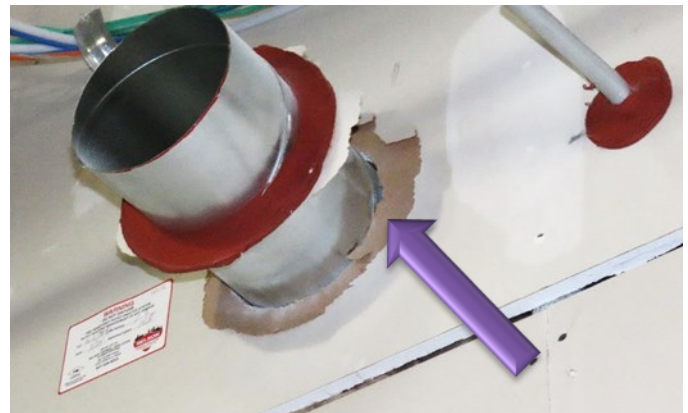
The round mechanical duct has been moved during the installation of the next component after the fire stopping was in-
