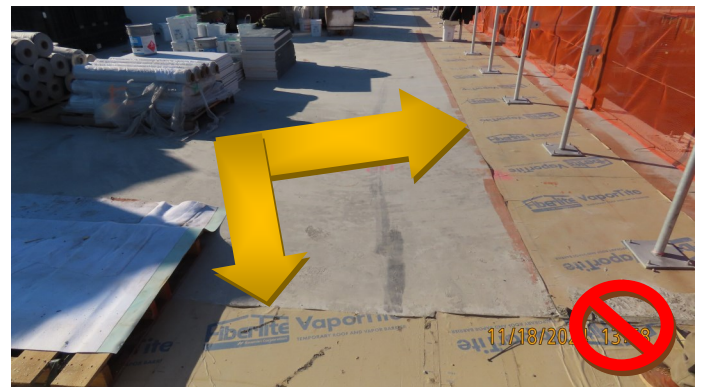
Roof vapor retarder is not sealed before the end of the day
