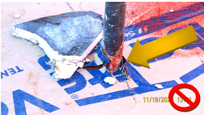
Roof penetration not sealed before the end of the day at the vapor retarder
